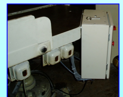
Electrical Cabinet placed on the back of the guillotine
